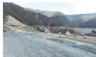
堤体盛立部での様子(全景) Embankment works at dam body (panoramic view)
