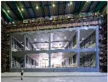
Keisei-Sugano under-pass road (the largest under-pass built with trenchless method in Japan)
